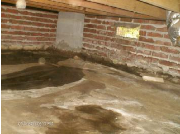
Moisture Penetration: (continued)
